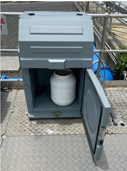
Figure 3. A refrigerated autosampler sampling inflow to a sewage treatment plant.
